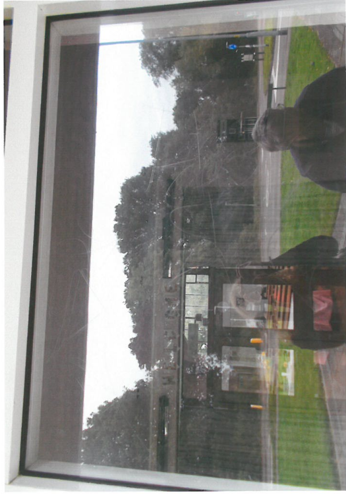
GRAFFITI on windows scratched on
