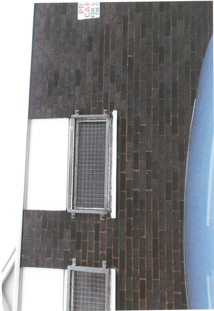
Grills on window to protect
